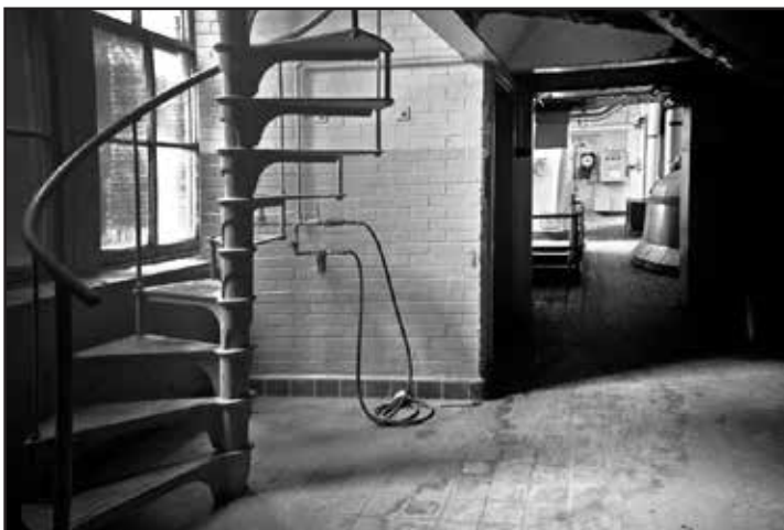
In the brewhouse between the preheating tank and kettle room. The spiral staircase goes into a kettle annex where a few smaller stainless steel kettles hide. If you looked right from this frame you would see the bottom of one of the kettles like the bottom of a steel mixing bowl.
