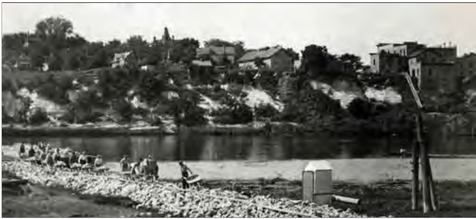
Constructing a wing dam on the Mississippi River. At top right, Banholzer brewery complex. 1905 image: MNHS.
